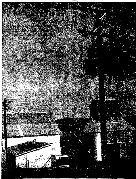
THE REA POLE with three transformers is becoming a more common sight each day as an increasing number of farmers add three-phase electric service to their farms. Warren Marotz, who farms northwest of Winside, uses the three-phase service to power his rolling mill and elevator. The elevator's 12,000-bushel capacity, built-in scales and pit and elevator facilities help make short work of feeding some 450 cattle.
